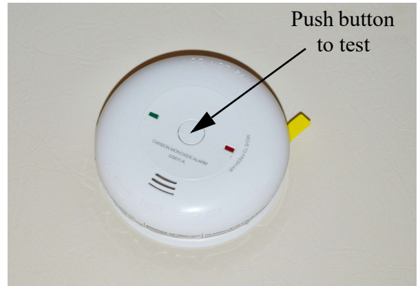
Carbon Monoxide Alarm
