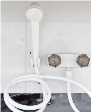
Exterior Shower/Wash Station -Typical View
